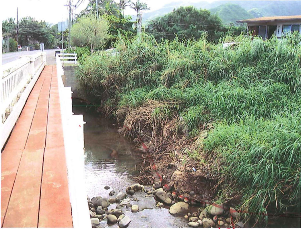
11. Kaipapa'u Stream Bridge – Looking to Kāne'ohe – After Storm 12-13-2008
